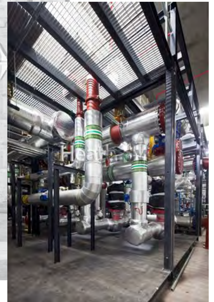
Duct supplying atmospheric air (denoted green on white)
