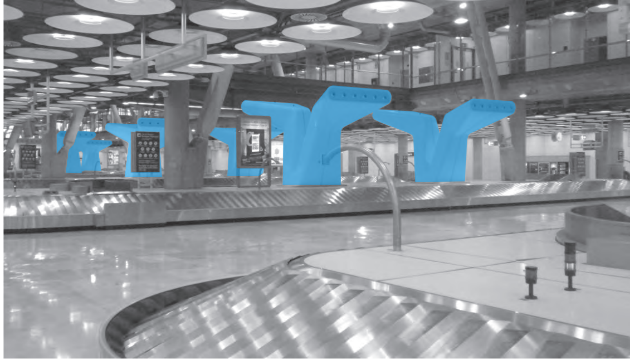
Displacement flow diffusers are located at check-in, baggage claim and security areas, which helps prevent air turbulence and draughts
