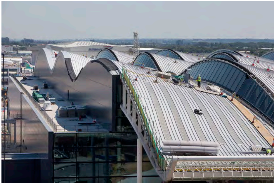
Glazing facing north to allow for comfortable daylight and to minimise heat gain
