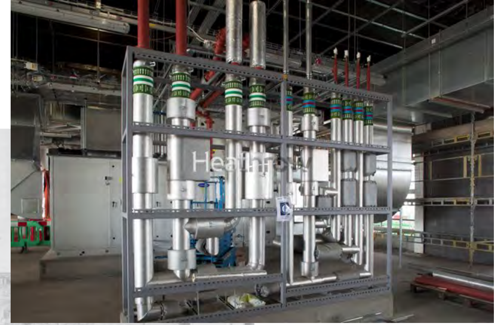
Pipe supplying atmospheric air (denoted green on white)
