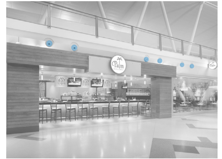
Jet nozzles along mezzanine edge of the concourse (high speed, low volume)
